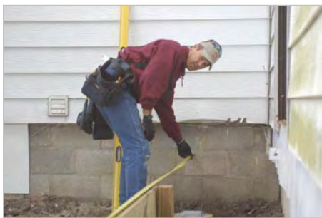
NARI member Mike Moore takes a measurement for the new deck on the back of the Bellis' home.
